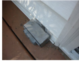
#2665 Loose Outlet Deck
