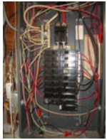
#2658 Interior Breaker Box
