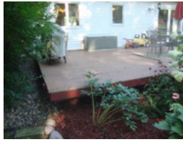
#2650 No Guard Rail Noted
