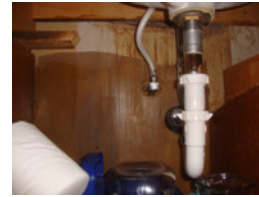
#2661 No Shut Off Valves
