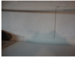
#2659 Stair Stepping Noted Rear Wall
