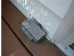
#2665 Loose Outlet Deck
