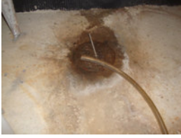
#2653 Corrosion Floor Drain
