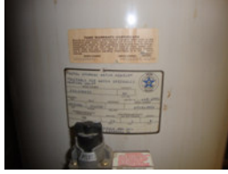
#2655 Older water Heater
