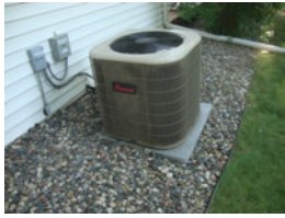
#2649 Air Cond. Needs Cleaning
