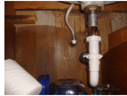
#2661 No Shut Off Valves
