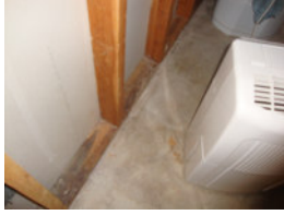
#2654 Stains At Framing
