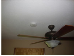
#2664 Smoke Detector Above Fan
