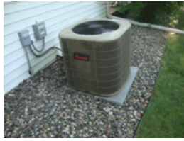
#2649 Air Cond. Needs Cleaning
