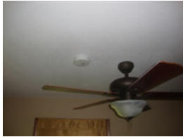
#2664 Smoke Detector Above Fan
