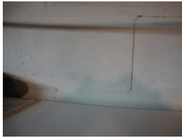
#2659 Stair Stepping Noted Rear Wall
